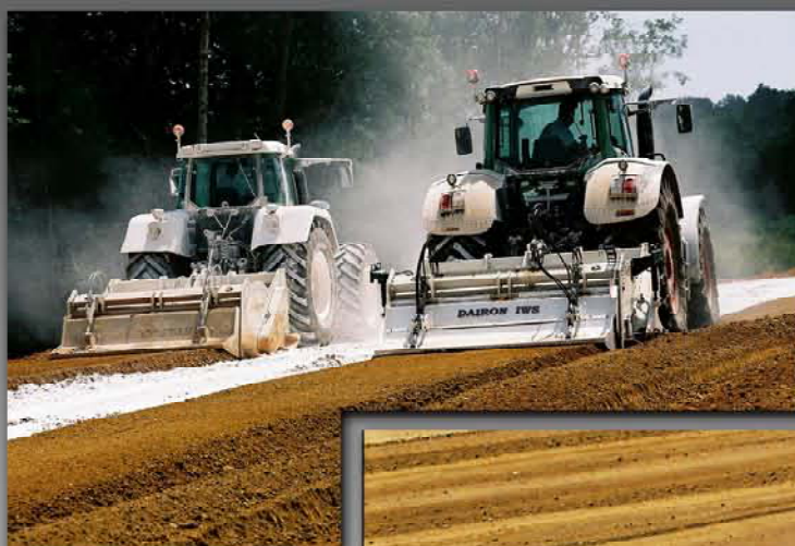
MSX 250 on site
